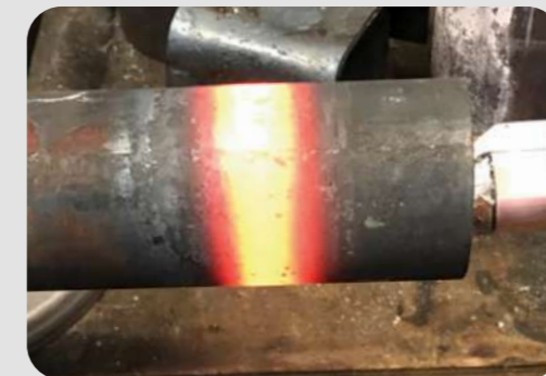
Gas boiler maintenance: - Heat Tube inductor S180/D50 - Powerduction 160LG
