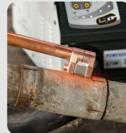
De-sealing an exhaust line assembly: - Small S90 inductor - Powerduction 37LG
